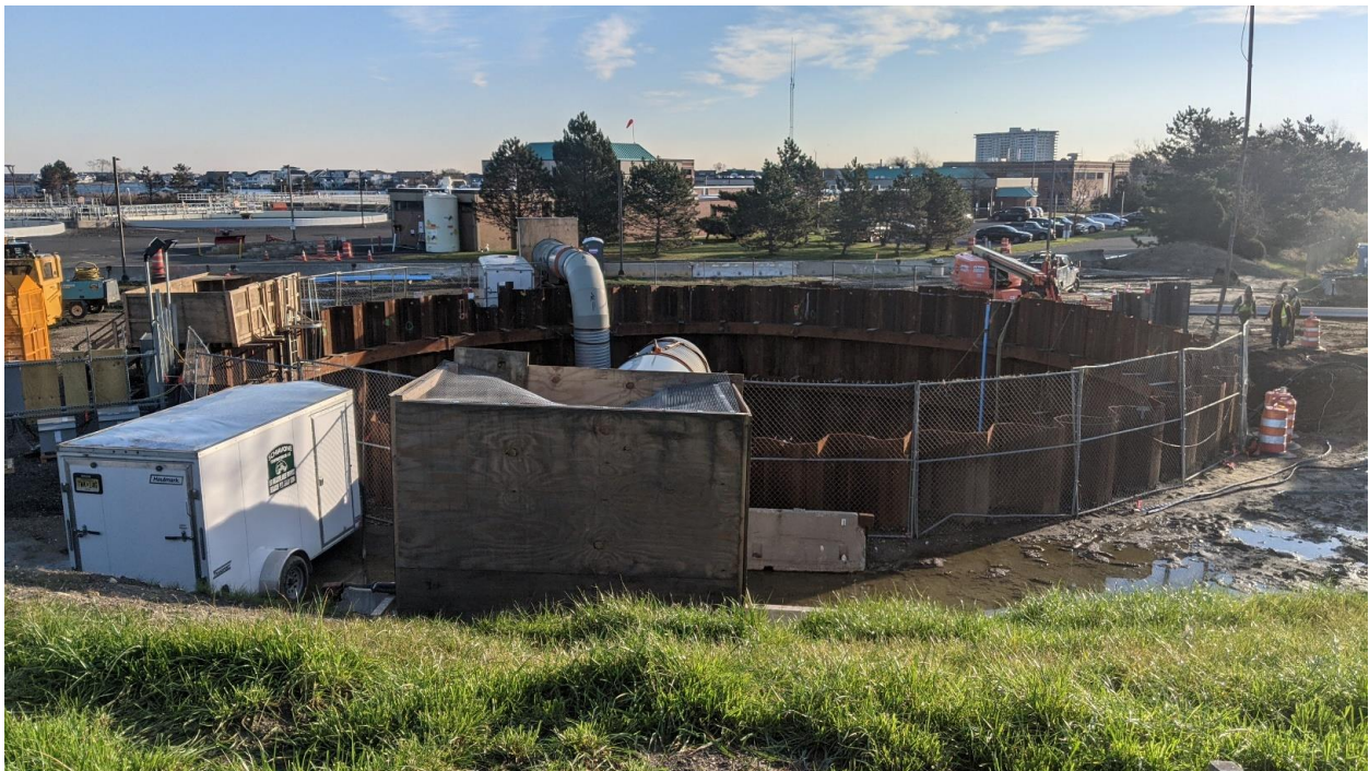
Excavation for the New Main Pump Station at the TRWRA Plant in Monmouth Beach
