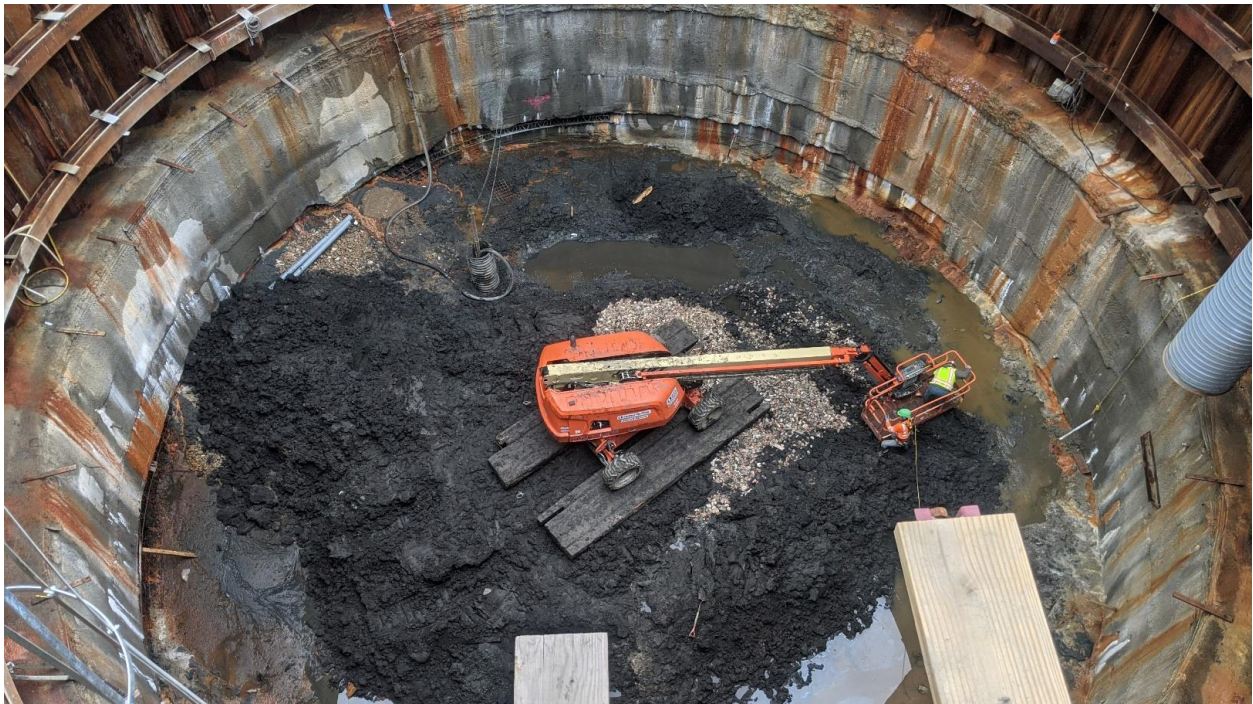
Excavation for the New Main Pump Station at the TRWRA Plant in Monmouth Beach
